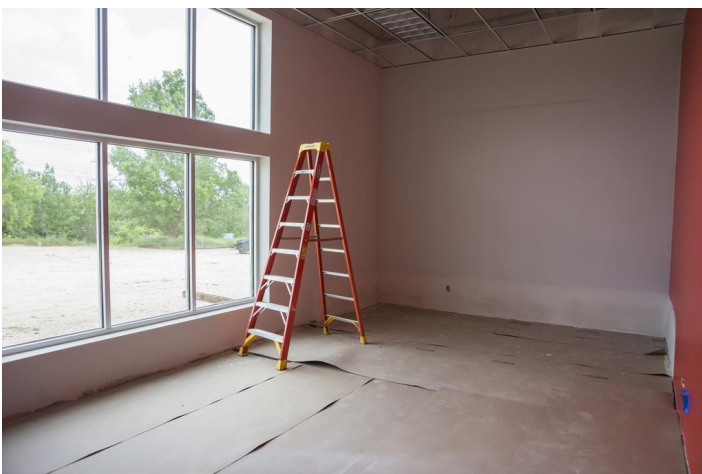
Structura Inc, an Austin-based construction company, is the general contractor for the project.
