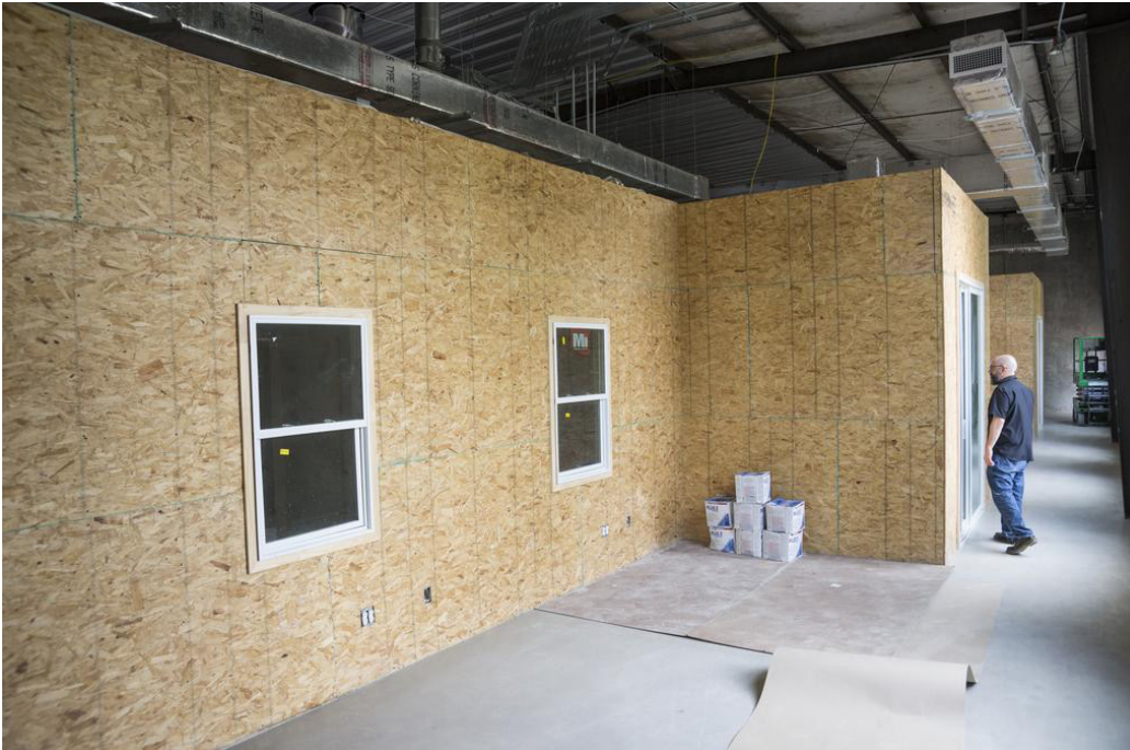
The architect is Stephen Oliver, principal of Opa Design Studio, which has a varied portfolio of residential and commercial projects including tenant build-outs for Kerbey Lane Cafe and Cuvee Coffee.
