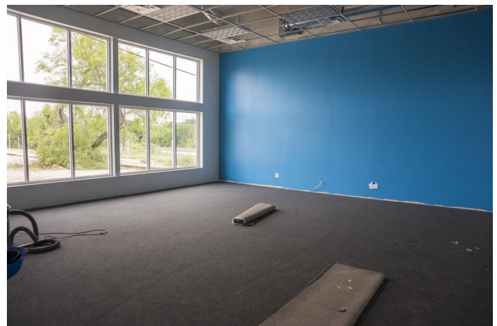
In the warehouse, large windows and garage doors have been installed to create wide streams of natural light and to allow the building to function as an indoor-outdoor space.
